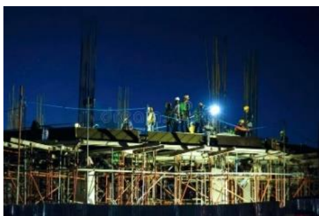
Fig.4.5 – Local task lighting
