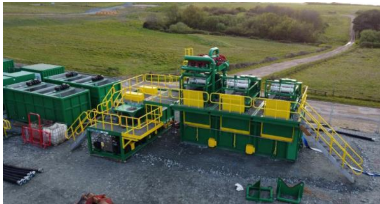
Figure 6.2: Drill Fluid Recycling Plant (typical)
