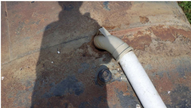
Photograph 1 – Compost effluent tank not overflowing and appeared to have spare capacity
