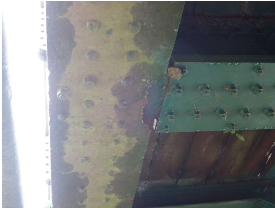
Photo 13: Loss of Section (28/08/2024)
