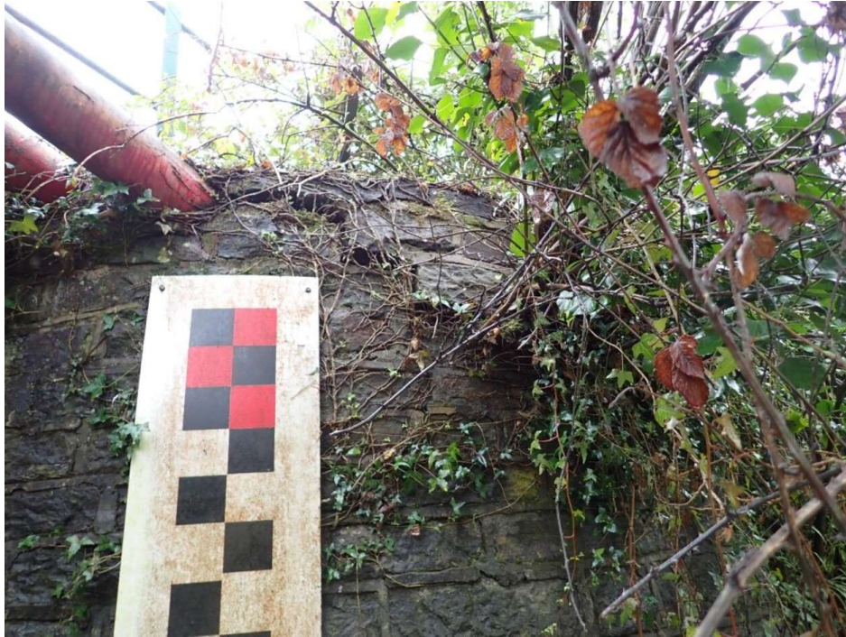
Photo 25: Displacement Around Tree (28/08/2024)
