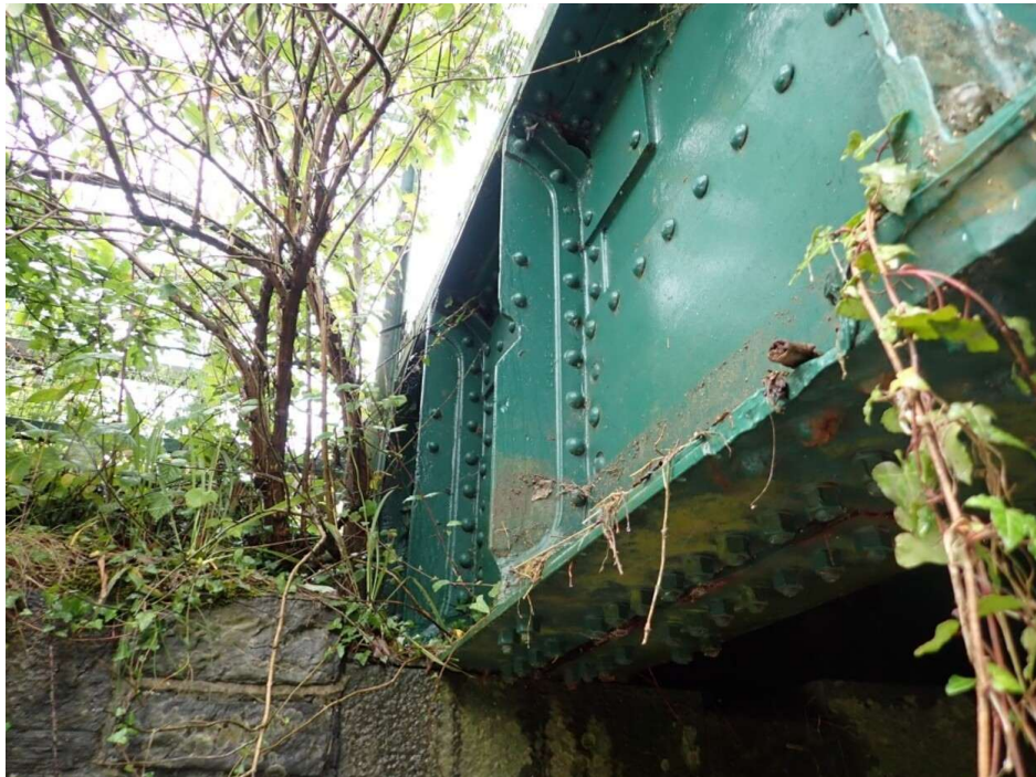
Photo 16: Typical Loss to Stiffeners (28/08/2024)
