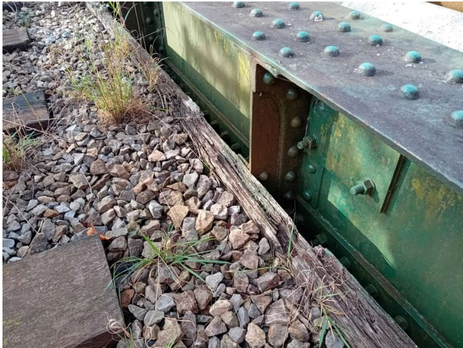
Photo 32: Upside Ballast Board (12/11/2024)
