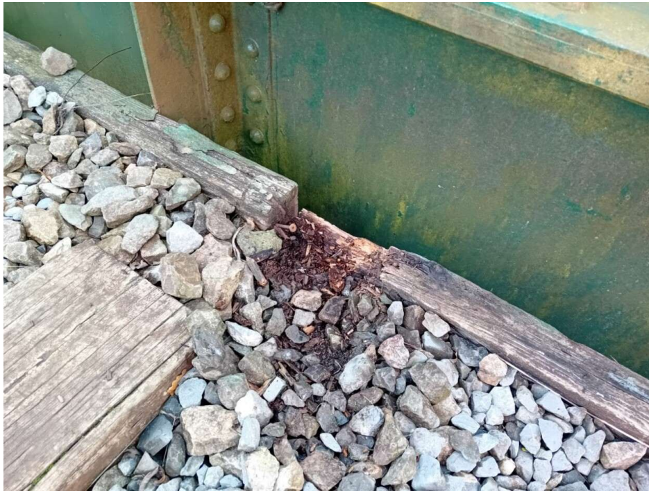
Photo 31: Downside Ballast Board (12/11/2024)
