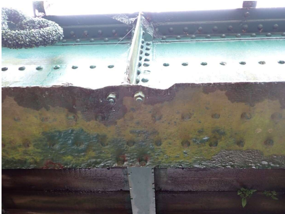
Photo 12: Loss of Section (28/08/2024)
