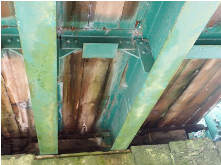
Photo 20: Typical Rail Bearer Corrosion. (28/08/2024)
