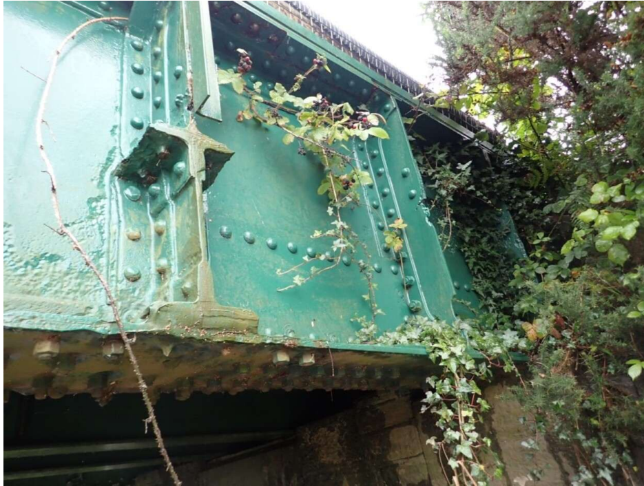
Photo 17: Typical Loss to Stiffeners (28/08/2024)
