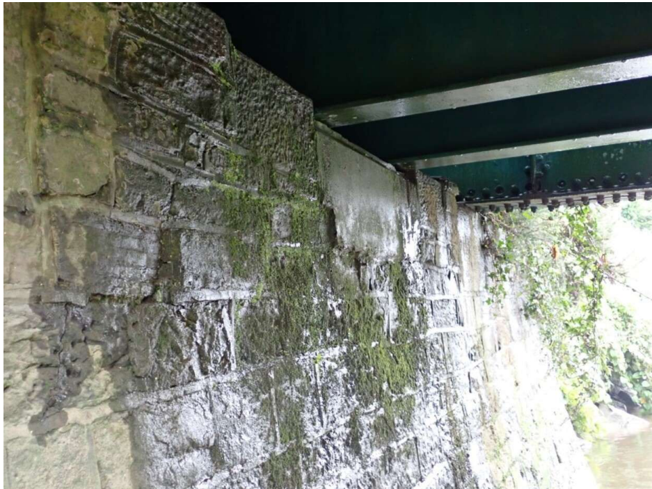
Photo 26: Loose to Hammer (28/08/2024)
