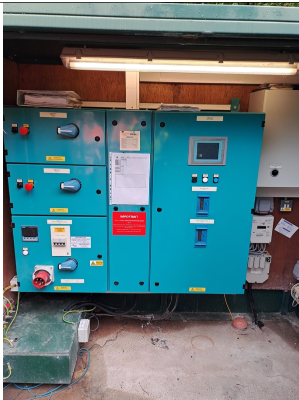
Figure 4 – The control box and panel as observed during the visit.
