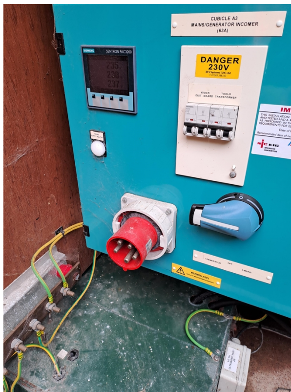
Figure 5 – The point where an external backup generator can be plugged in.
