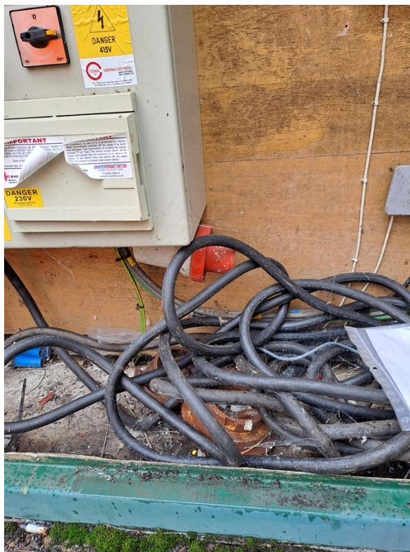
Figure 6 – The mobile backup generator point in place.
