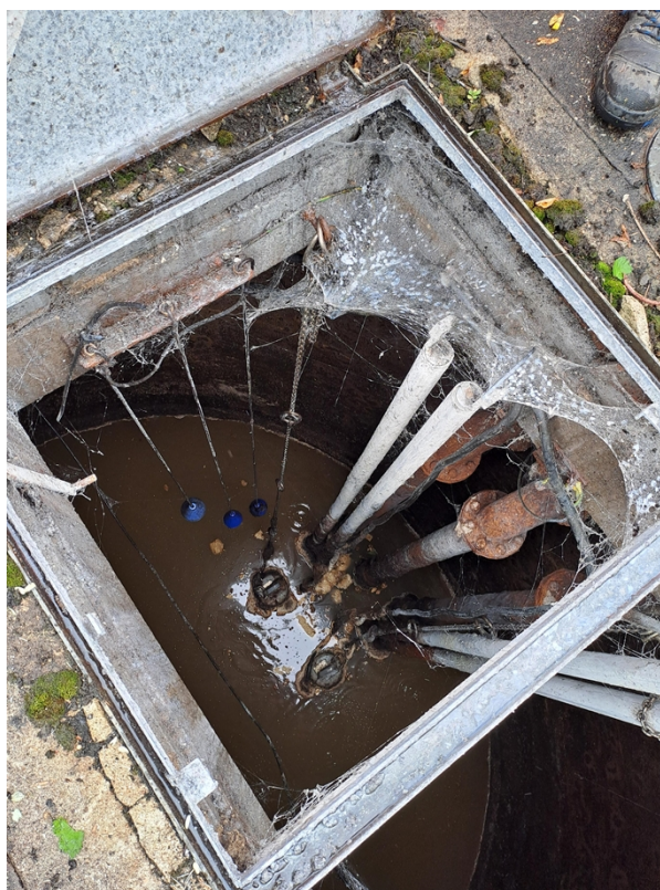
Figure 3 – The condition of the wet well as observed during the visit.
