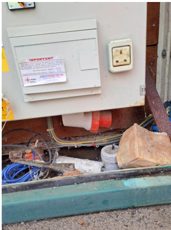
Figure 6 – The mobile backup generator plug in point in place.
