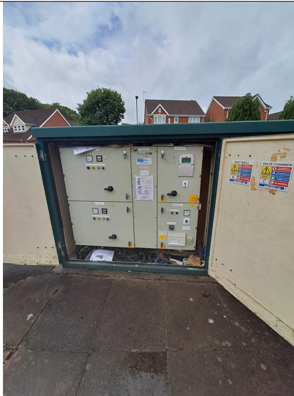
Figure 5 – The control box and panels as observed during the visit.
