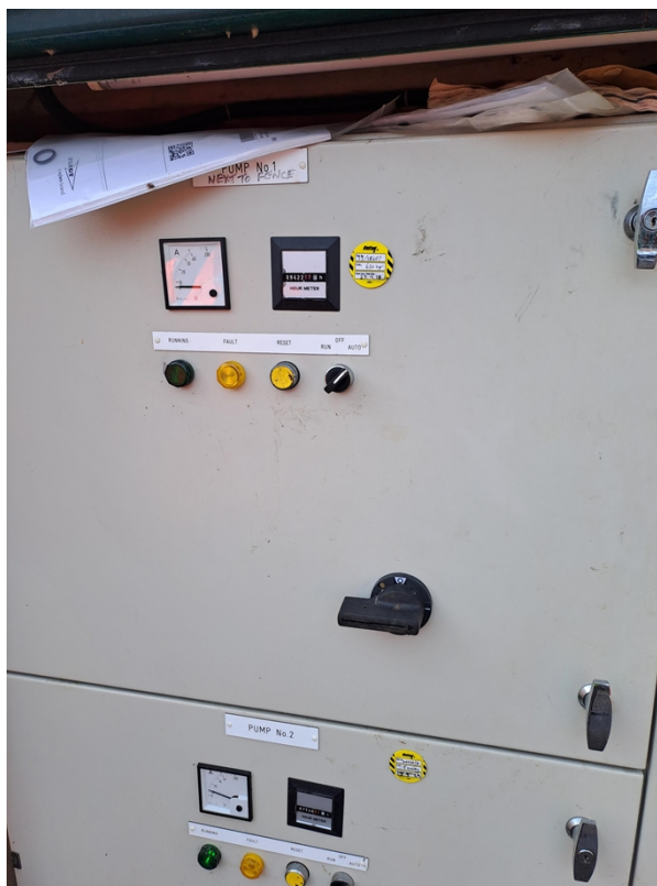
Figure 7 – The control panel with the power off and isolator functions present.
