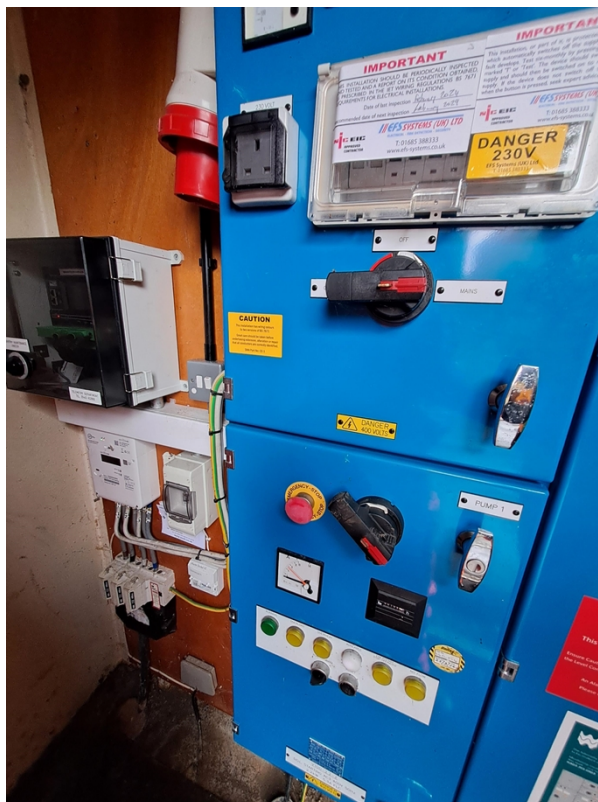
Figure 7 – The emergency stop function and backup generator point in place as observed during the inspection.
