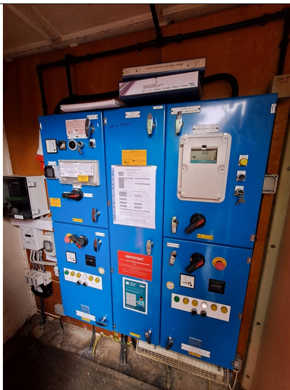
Figure 6 – The control panels and systems as observed during the visit.
