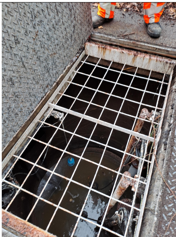
Figure 3 – The wet well where telemetry systems can be seen.
