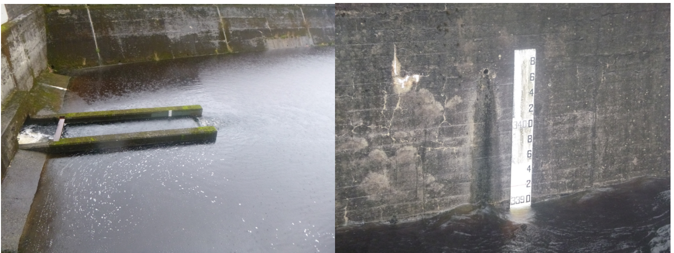
Figures 1 & 2: Staff Gauges at Nant y Moch Reservoir
