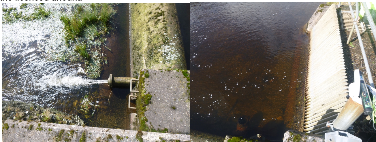
Figures 9 & 10: Orifice Plate and Abstraction Screen at Afon Llywernog
