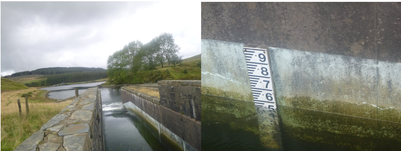
Figures 5 & 6: The outfall and Staff Gauge at Afon Castell
