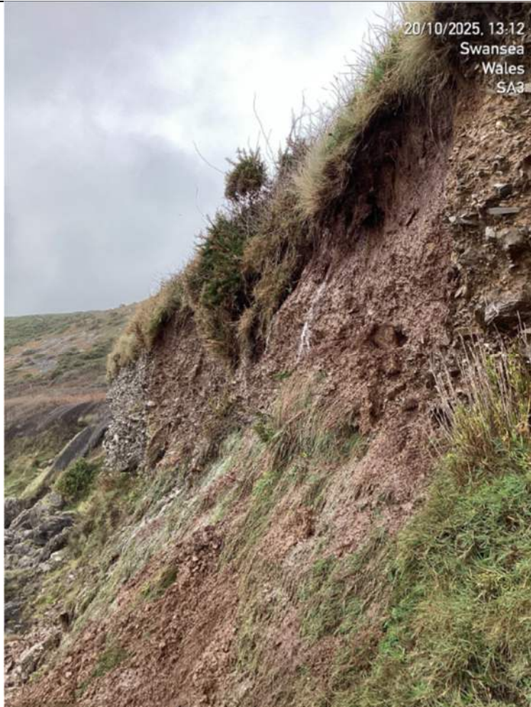
Flow emanating from the footpath bifurcated/filtered through sub-soil, leaching out as seen above.
