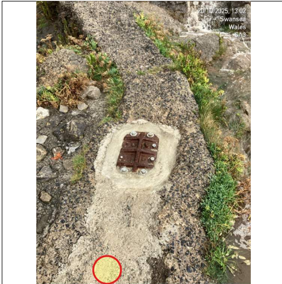
Hatch-plate d/s from discharge on footpath. The highlighted spot indicates where the metal sampling pot was wedged in the line (approx. 1m d/s from plate)
