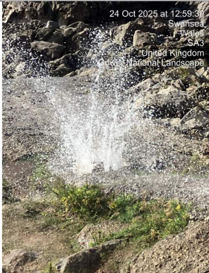
Once the pumps were switched back on, discharge escaped from the hatch due to lack of hermetic sea
