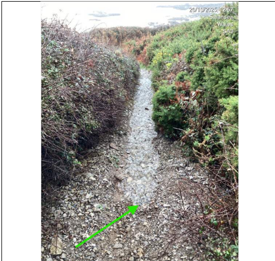
W3W ///sometimes.flown.package Effluent has backed-up the line due to obstruction (metal sampling pot) and has discharged from the nearest weak-point in the network
