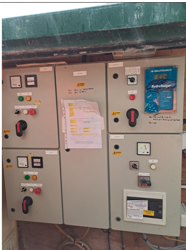
Figure 5 – The control panel as observed during the visit.
