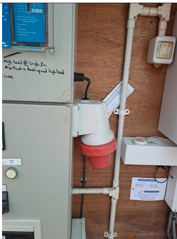
Figure 6 – The mobile generator plug in point as observed during the visit.
