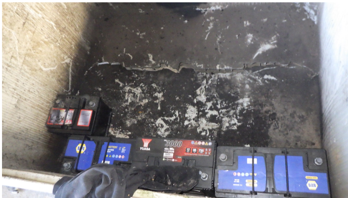
Batteries storage box
