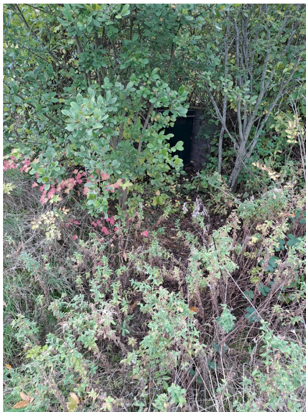
Figure 2 – The condition of the system control box access as observed during the visit.
