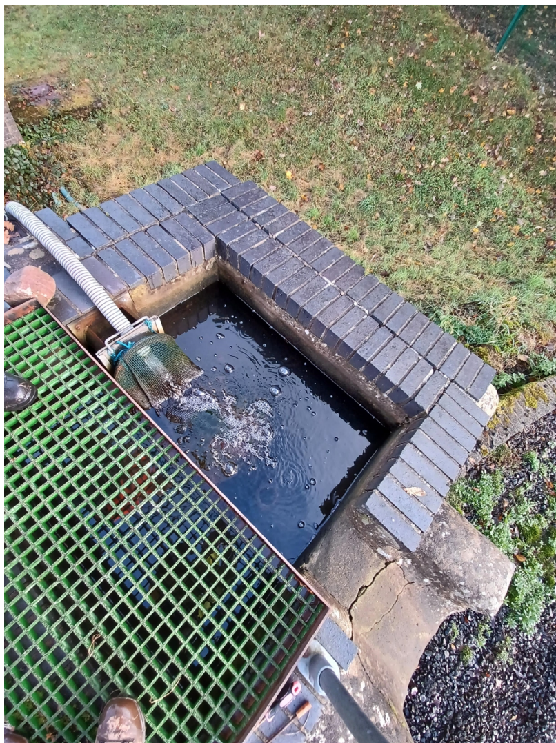
Image 1: Pipe outlet from pump well with copa sack on end.
