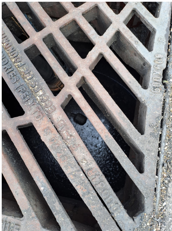
Figure 3 - The sump/separator conditions as observed during the visit.
