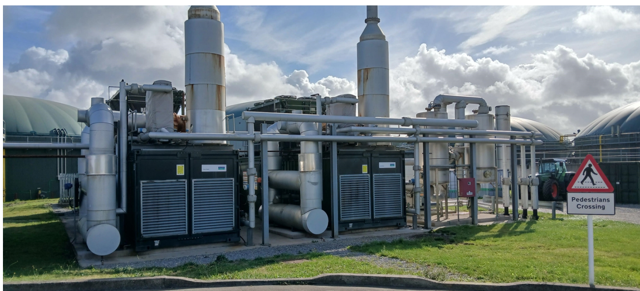
Photo 1 - CHP engines at Severn Trent Parc Stormy
