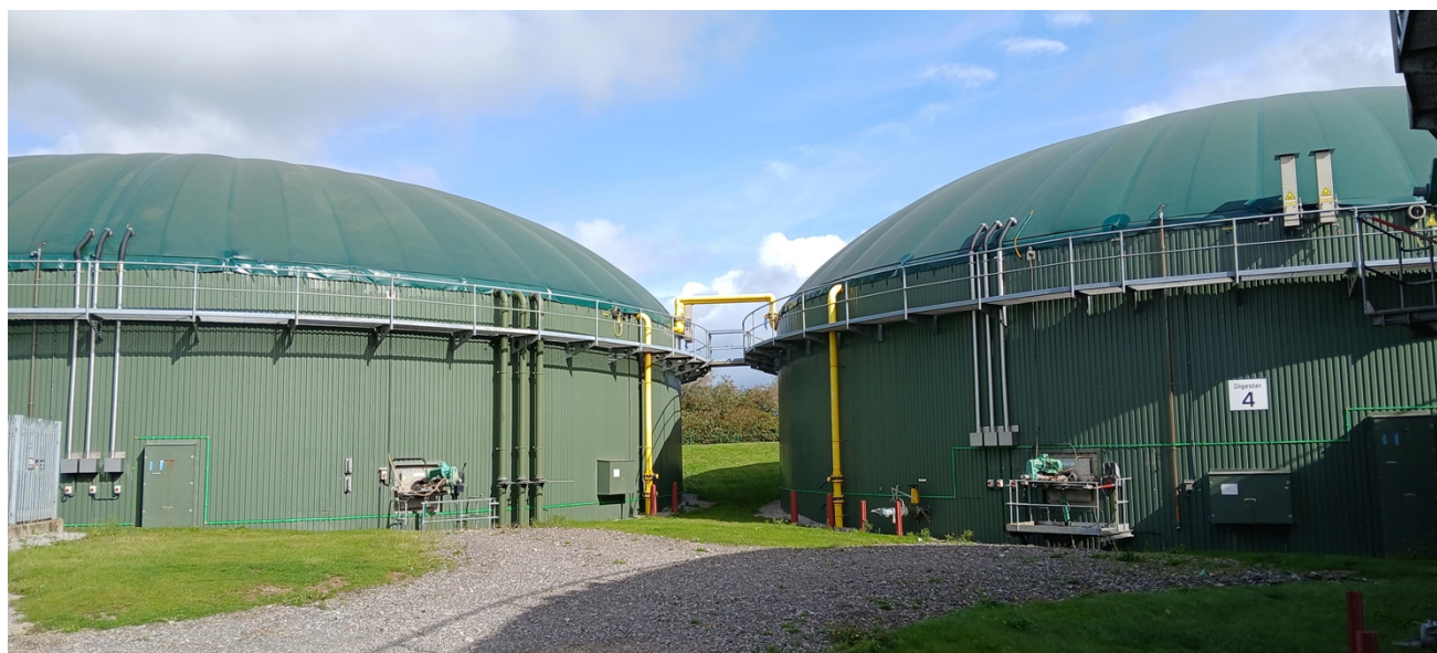
Photo 4 - Digester Units at Severn Trent Parc Stormy
