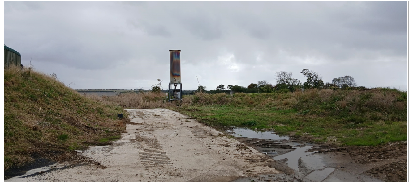
Photo 3 - Gas flare at Pancross Farm
