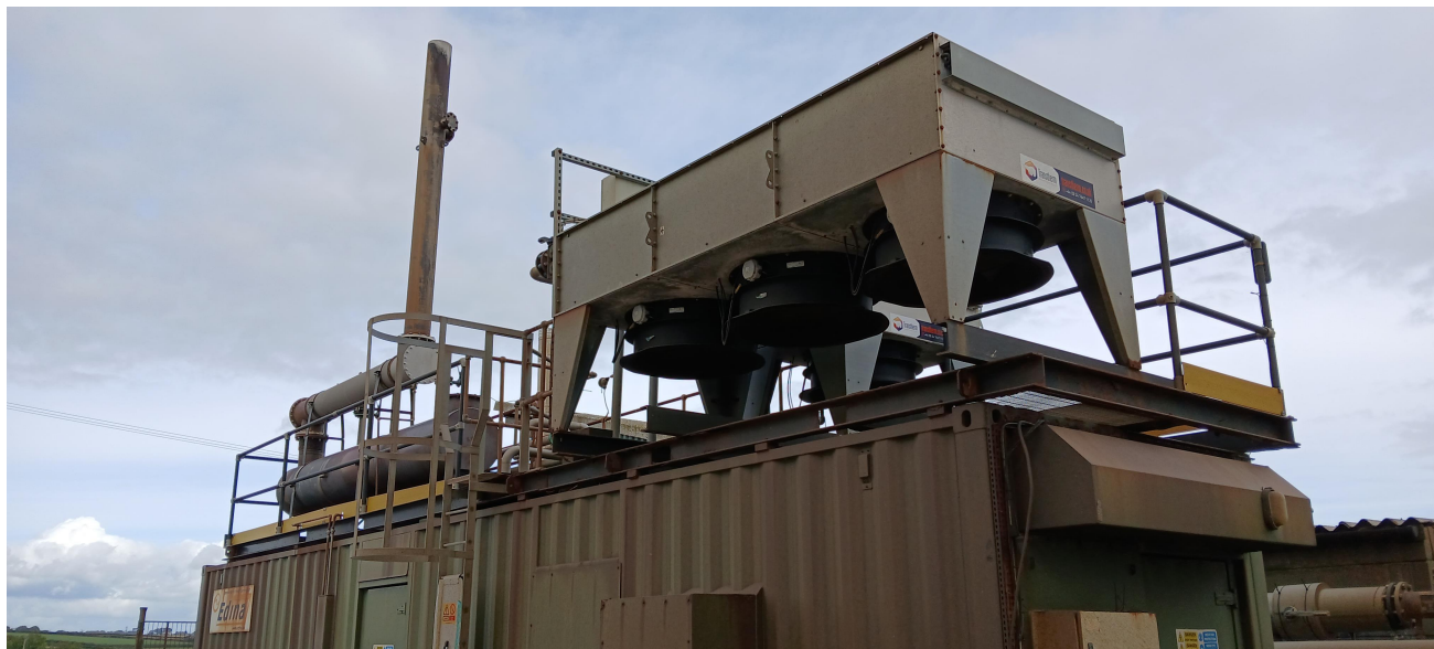
Photo 1 - CHP engine at Pancross Farm
