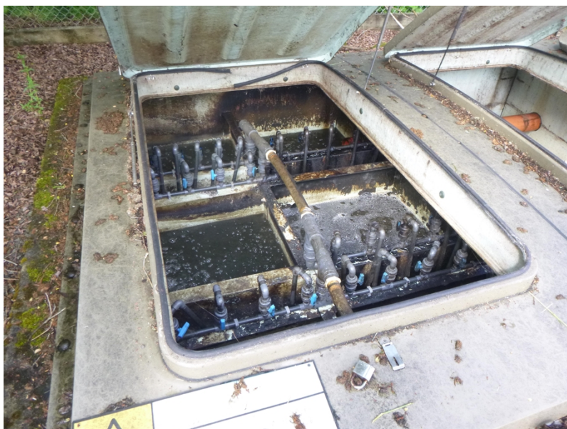
Photograph 3: Biological Aerated Filter (BAF)
