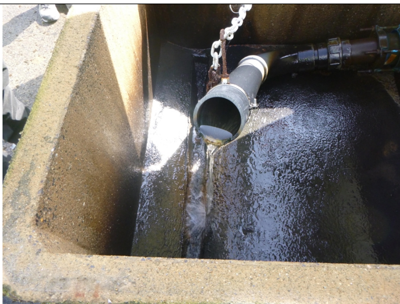
Photograph 7: Discharge from reedbed
