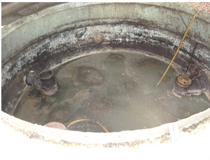
Photograph 1: Inlet tank used for primary settlement
