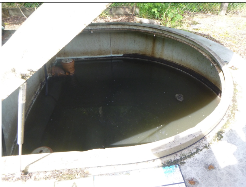
Photograph 4: Secondary settlement tank
