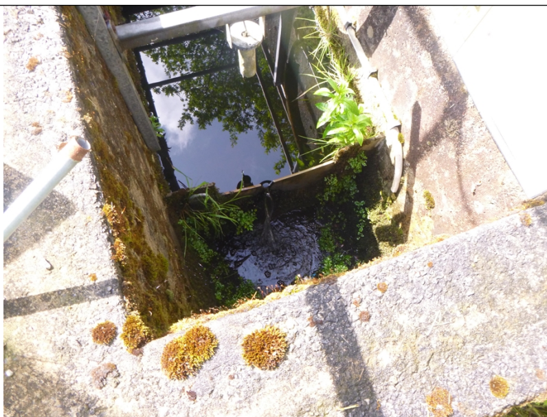
Photograph 9: Final effluent sampling point
