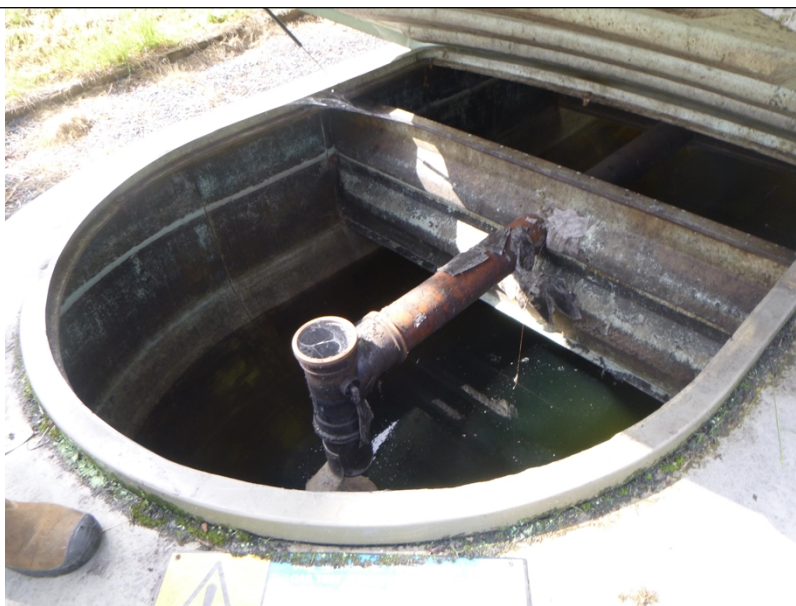
Photograph 2: Sludge holding tank
