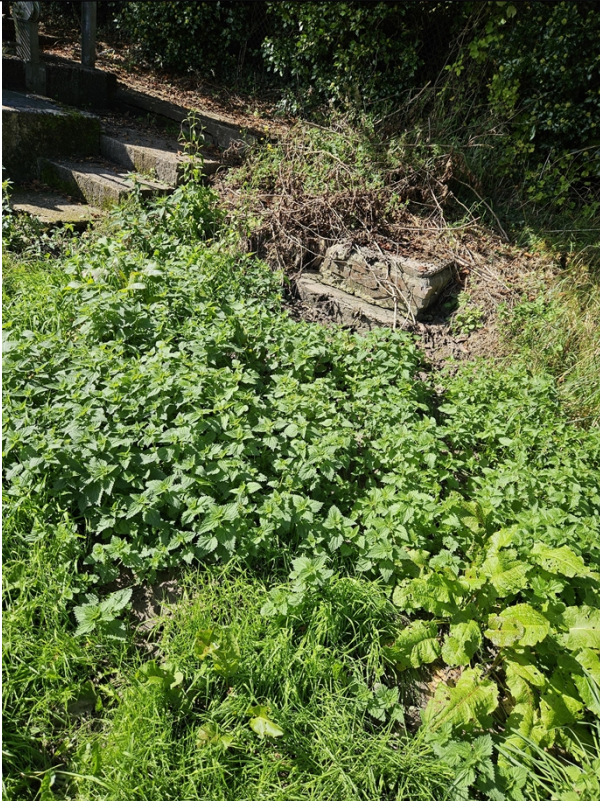
Evidence of spill from manhole at the inlet.
