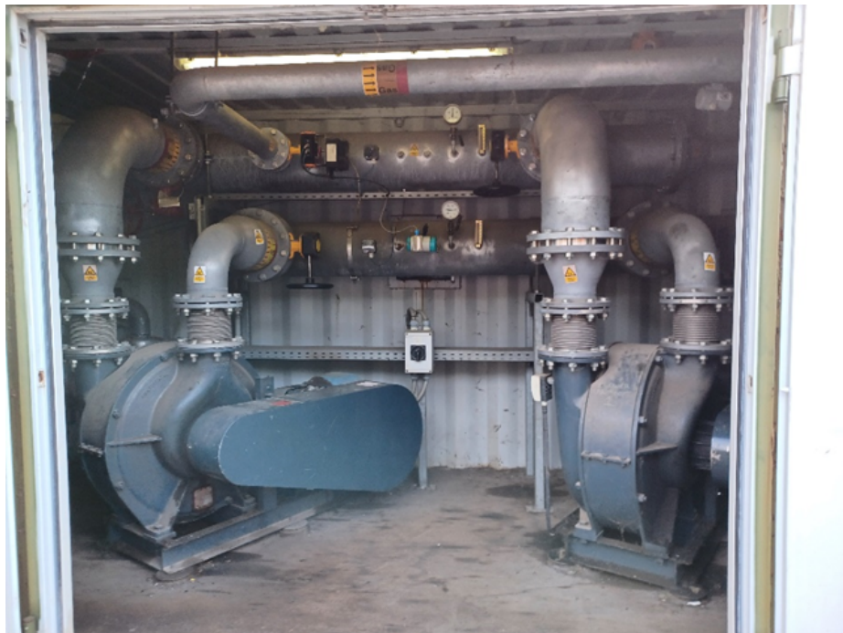
Image 1: View of Booster Room
