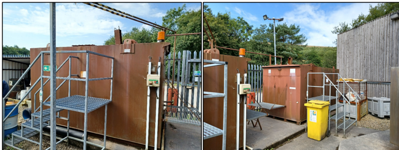
Image 4: Integrated oil storage vessels onsite - clean (left) and dirty (right).
