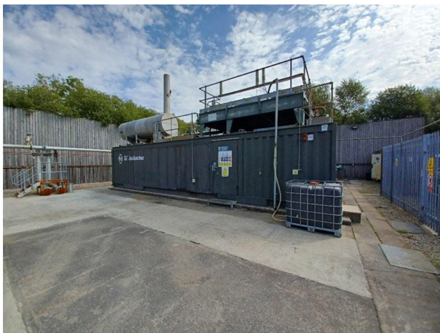
Image 2: View of Jenbacher 320 engine
