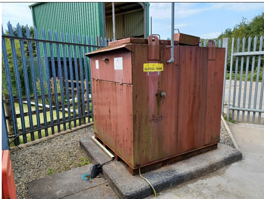
Image 5: Integrated glycol storage tank
