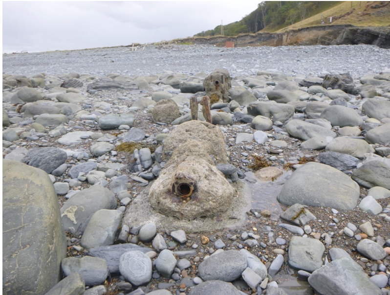
Photograph 4: Broken pipework on Tanybwllch Beach at SN 57703 79658
