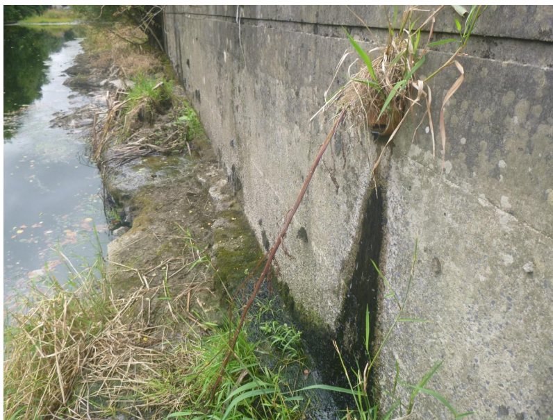
Photograph 1: Derwenfa's final effluent outfall
