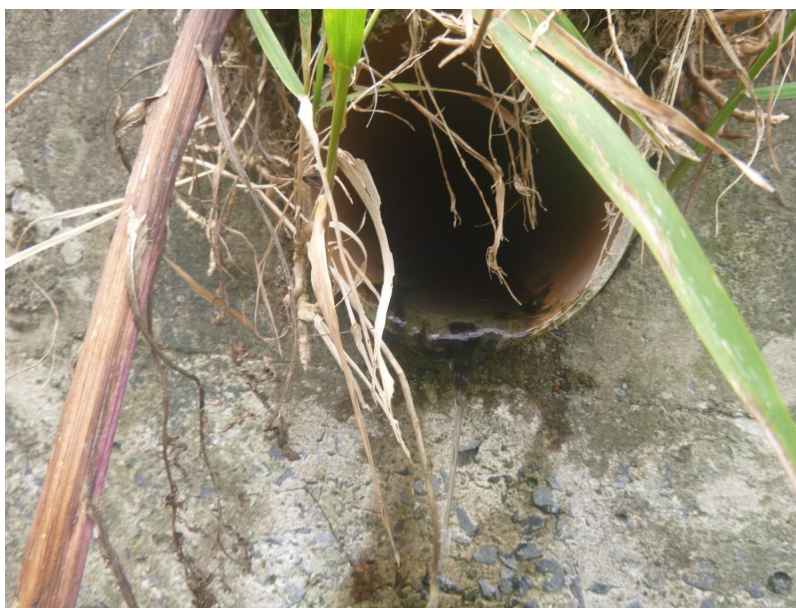
Photograph 2: Derwenfa's final effluent discharge pipe containing traces of sewage fungus
