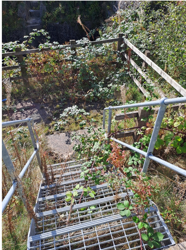
Figure 7: The access route to the sample/discharge point as observed during the visit.
