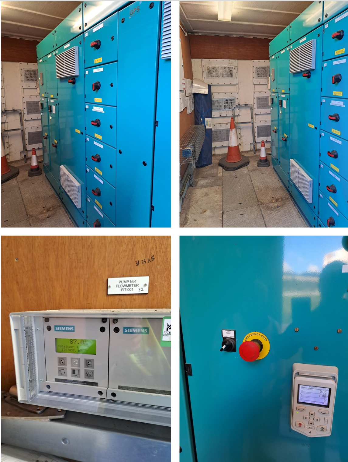
Figure 6: The control room infrastructure as observed during the visit.
