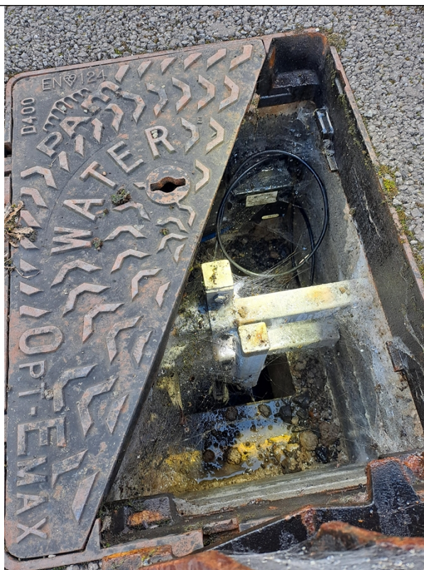
Figure 4: The telemetry and EDM sensors as observed during the visit.
