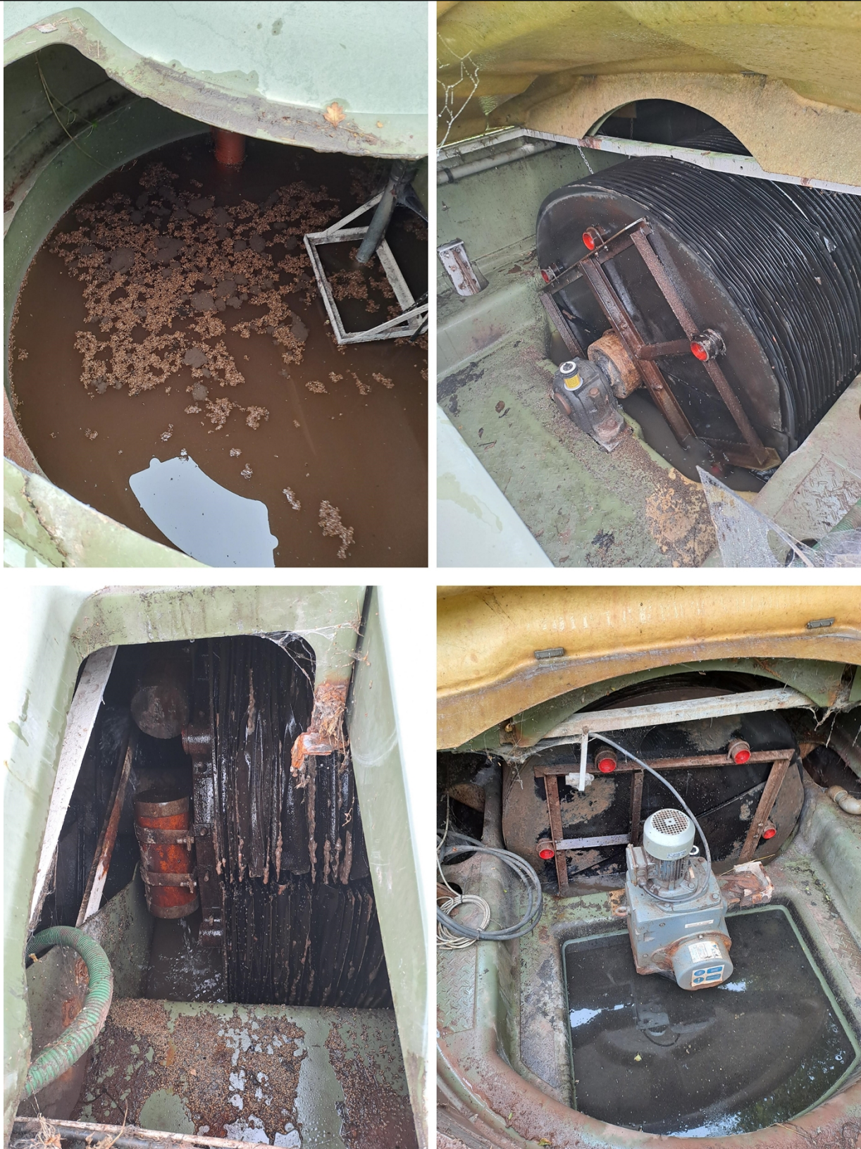
Figure 4: The treatment system chamber as observed during the visit.
