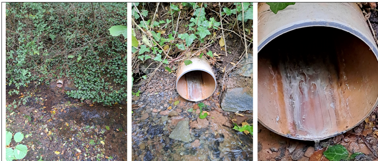
Figure 2: The discharge/sample point as observed during the visit.
