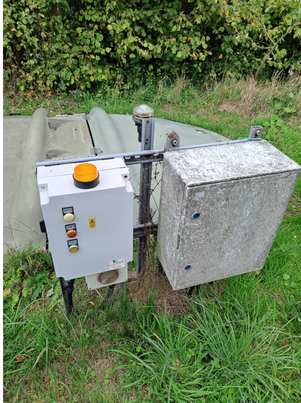
Figure 5: The control box as observed during the visit.
