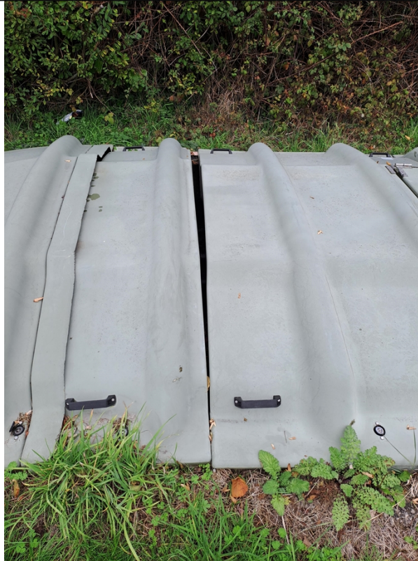
Figure 3: The treatment system with a small gap in the cover as observed during the visit.
