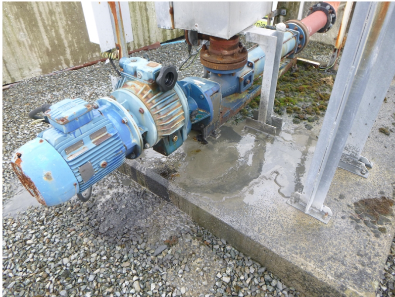
Photograph 4: Small leak evident in sludge pump
