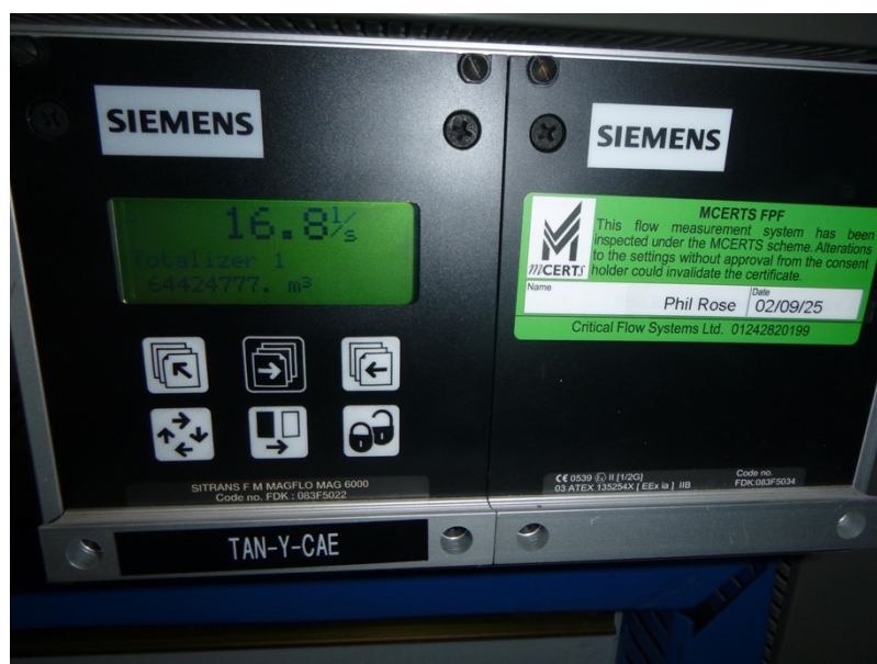
Photograph 1: Visual display for Tan y Cae SPS MCERTS FPF meter
