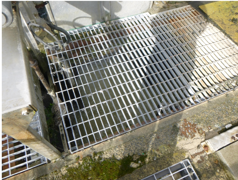
Photograph 2: Aberystwyth STW inlet and UWWTD crude sewage sampling point
