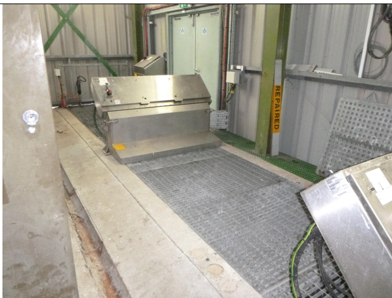
Photograph 7: One of two UV banks
