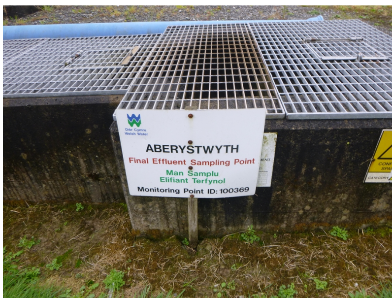
Photograph 10: Final effluent sampling point
