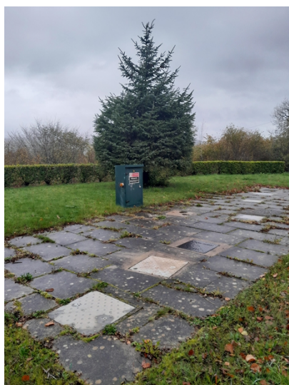
Package Treatment Plant (Fig 1)
