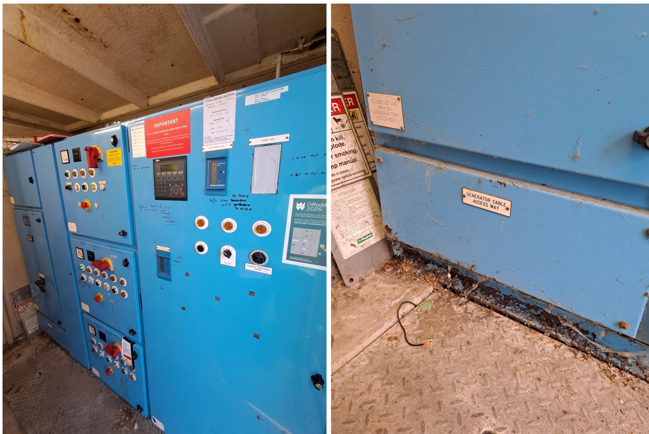
Figure 1: The control room as observed during the visit.
