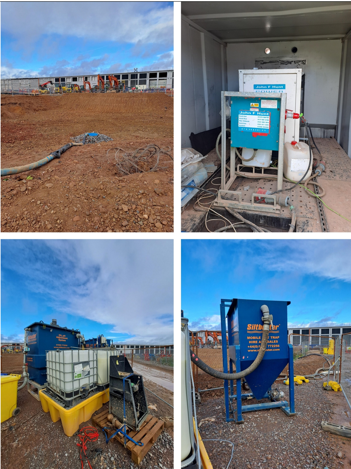
Figure 3: The treatment system infrastructure as observed during the visit.
