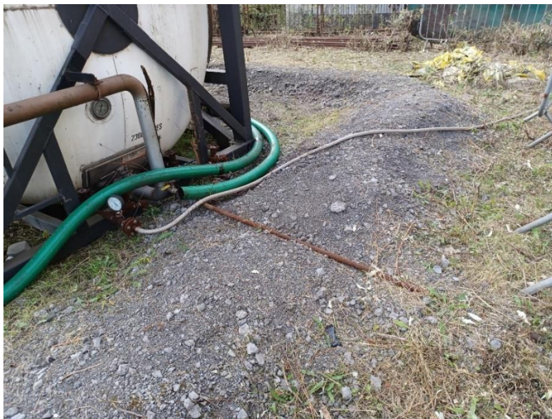
Image 4: Small offtake pipework from the outlet of the back-up oil tank, seen to discharge into the North Tank earth bund.
