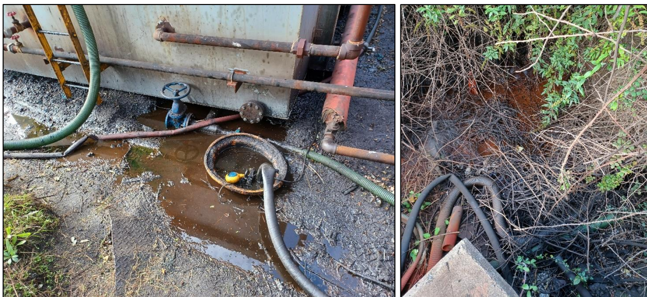
Images 6 & 7: Sump within the tertiary containment area, outlet observed as entering ditch to rear of the bund.
