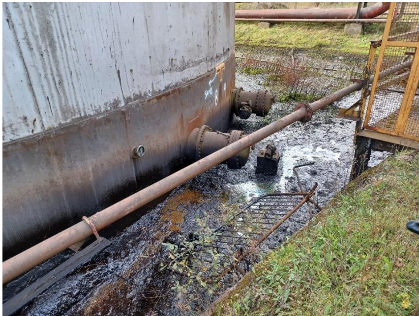
Image 2: Accumulation of hydrocarbon contaminated sludges (visual perspective) around the north-western face of the South Tank
