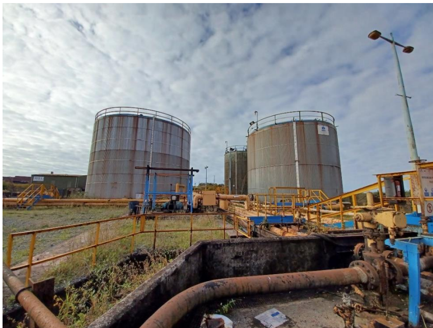
Image 1: View of the Pheonix Oil Tank Farm
