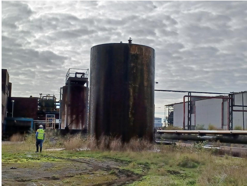
Image 9: Overflowing tank associated with Energy Department
