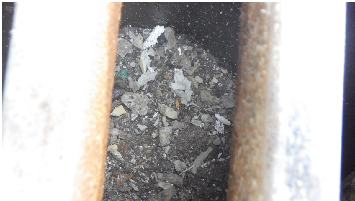
Residue at the bottom of surface drain.
