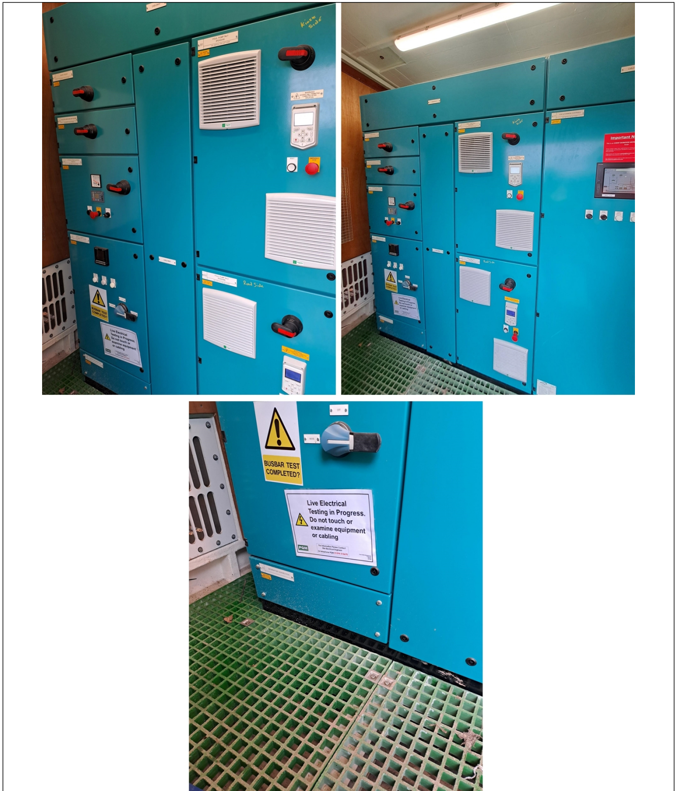
Figure 2 – The control panel and associated infrastructure as observed during the visit.
