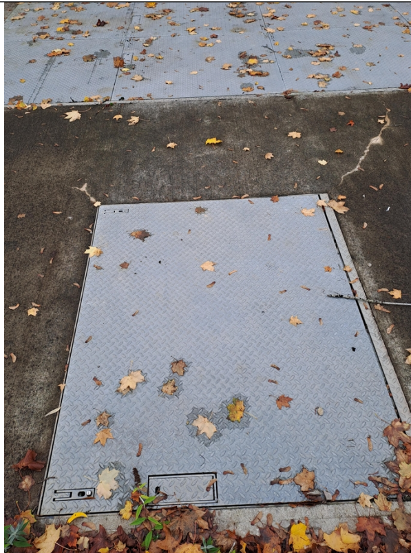
Figure 5 – The sample point chamber which was not able to be lifted at the time of the visit.
