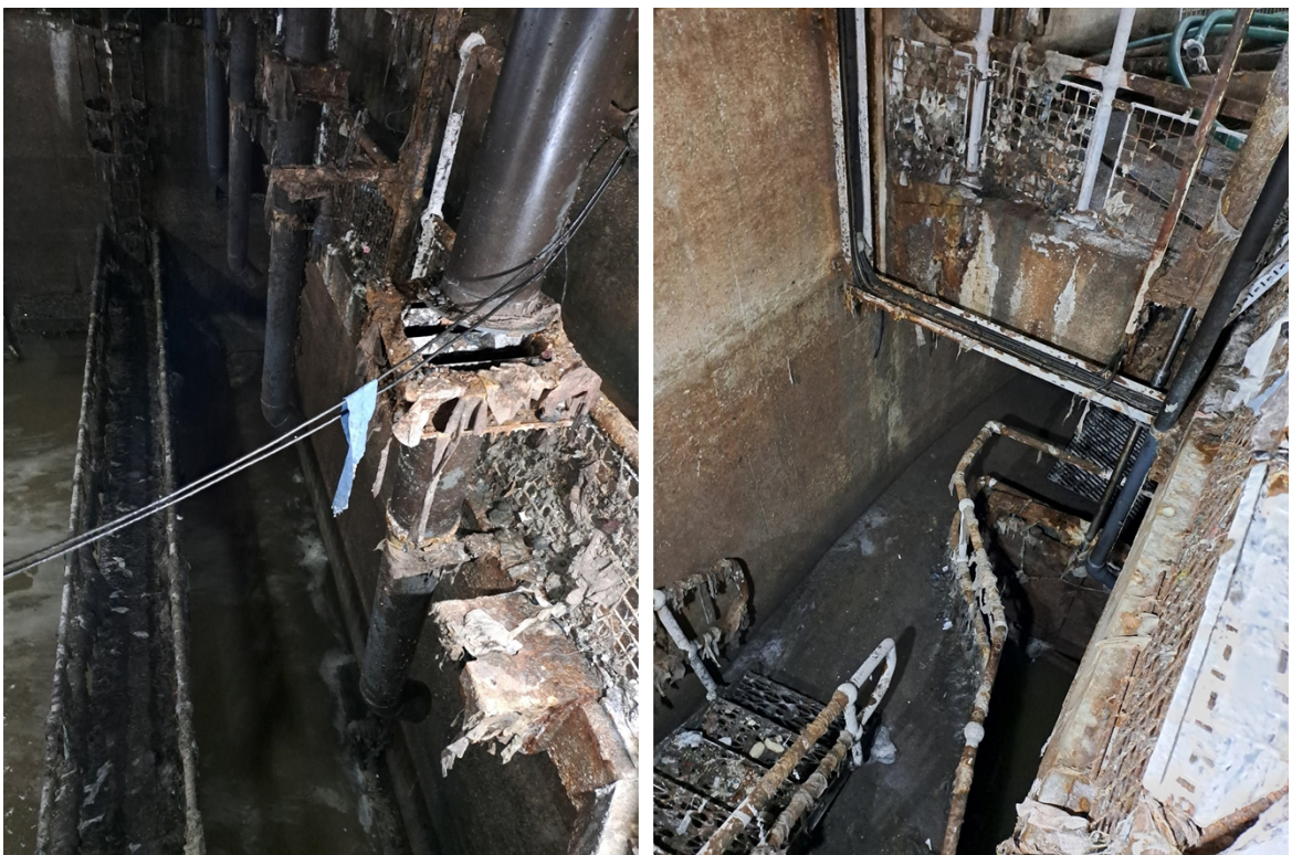
Figure 6 – The rag build up as observed during the visit.
