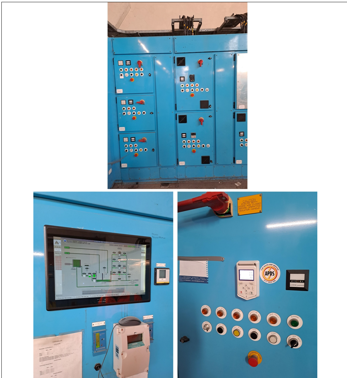
Figure 2 – The control panels and readouts as observed during the visit.
