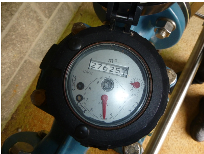
Photograph 5: Meter at Point C
