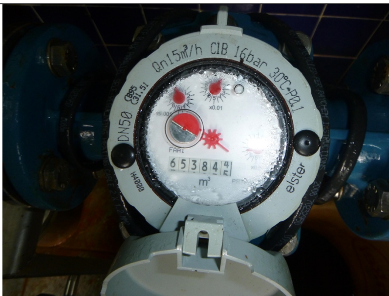
Photograph 4: Meter at Point B
