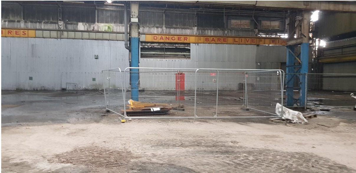
Figure 7 – Western facility boundary wall requiring concrete block protection.
