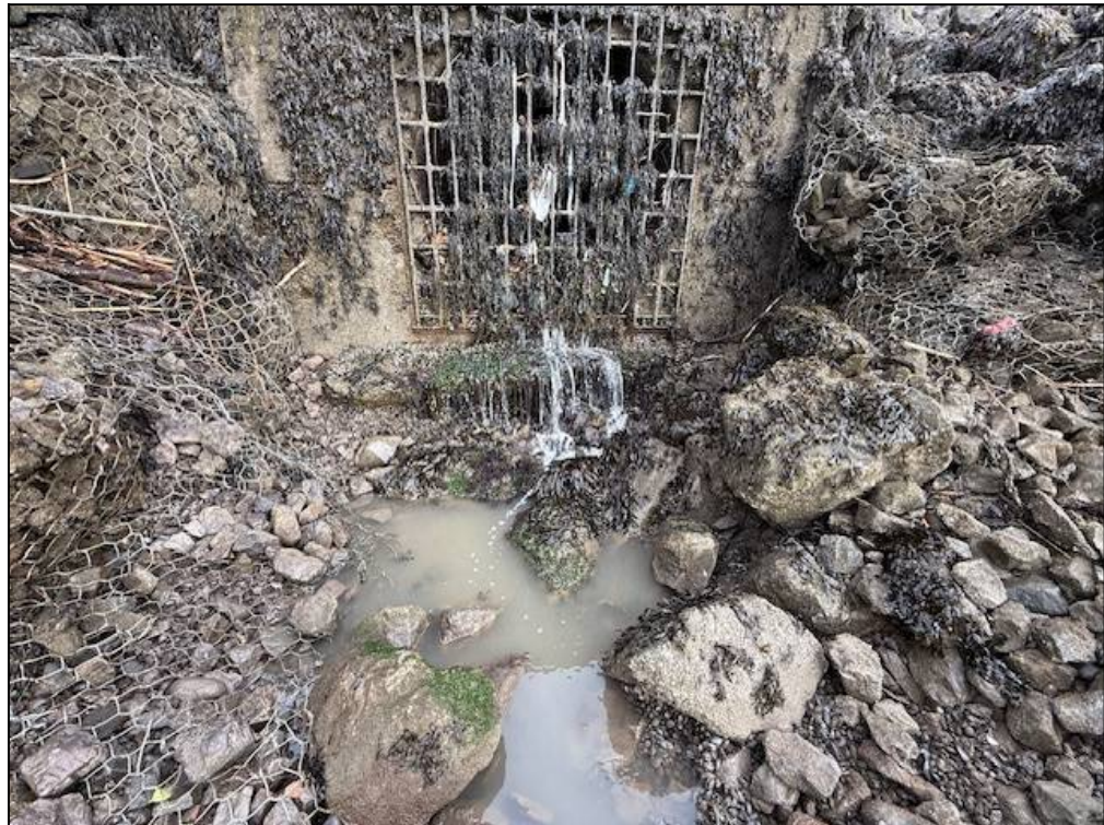
IMAGES OF DAMAGE TO THE EXISTING OUTFALL - WING WALLS, APRON & GRATING
