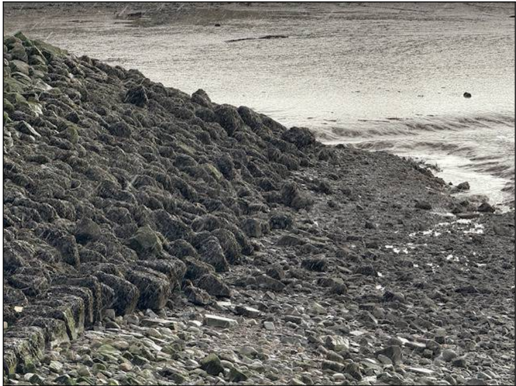
IMAGES OF DAMAGE TO THE TOE AND APRON OF THE EXISTING ROCK REVETMENT
