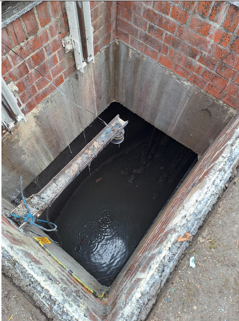
Figure 4 – The telemetry sensor as observed at the time of the visit.
