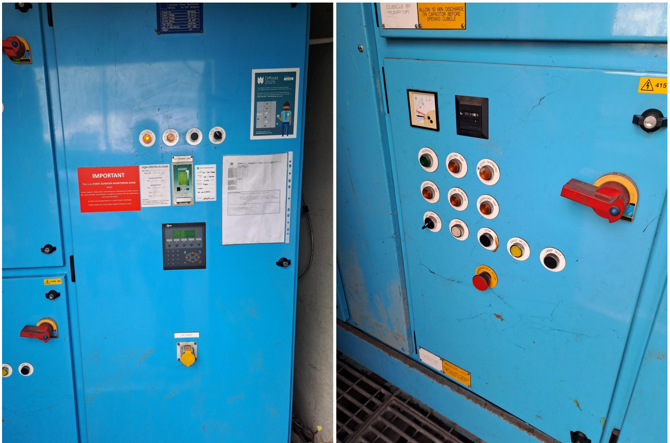
Figure 6 – The control panel as observed during the visit.
