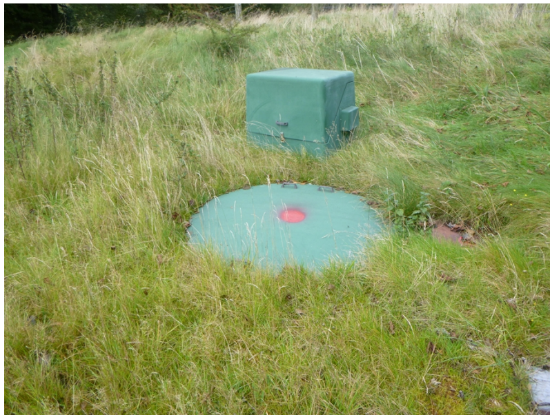
Photograph 1: Sewage treatment system
