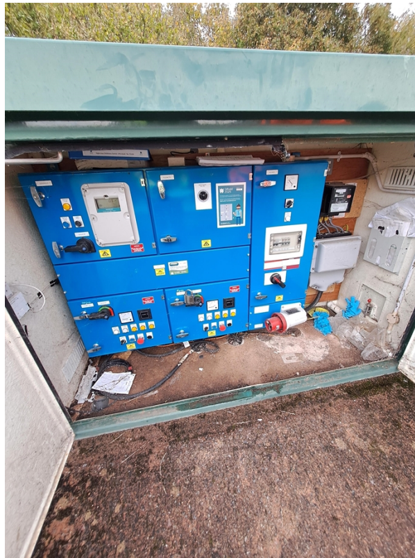
Figure 2 – The control box as observed during the visit.
