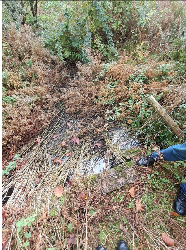
Figure 7 – The headwall located at ST2831088173, within 10m of the suspected discharge point as it appears on the NRW mapping system.
