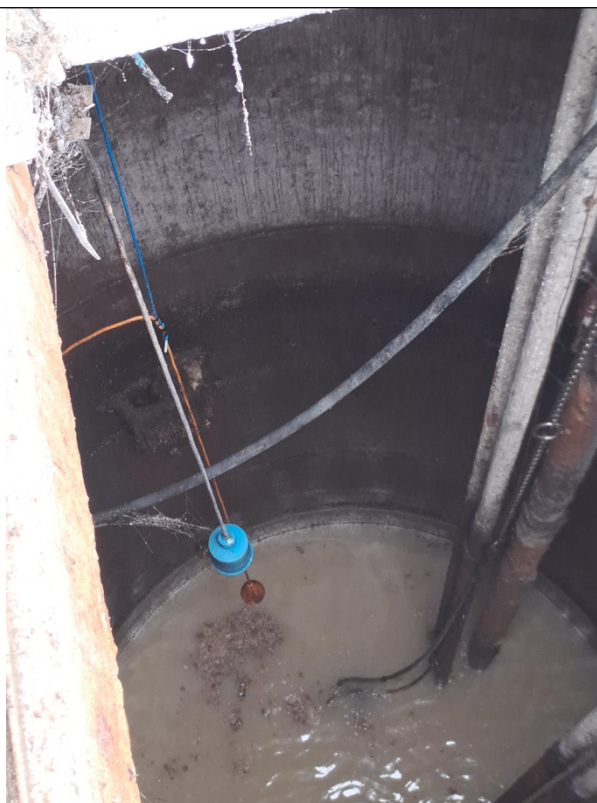
Figure 4 – The telemetry sensor heads as observed during the visit.
