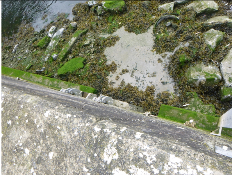
Photograph 7: Possible unpermitted storm overflow on incoming sewer network
