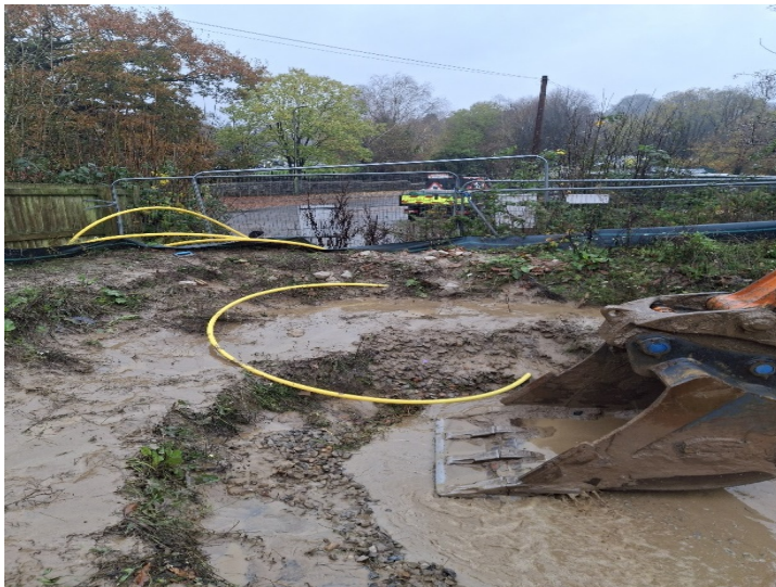
Figure 3: Location where silt mitigation failed and silt discharge occurred
