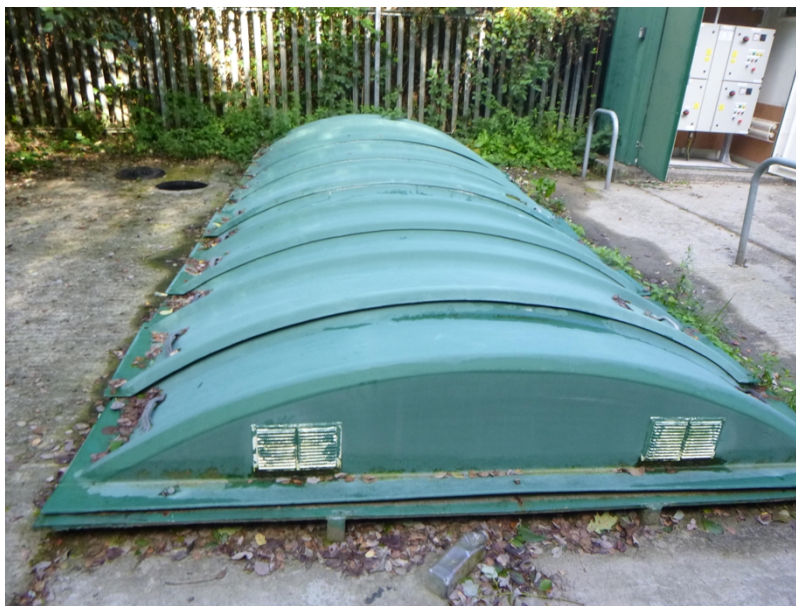
Photograph 1: Rotating Biological Contractor (RBC)
