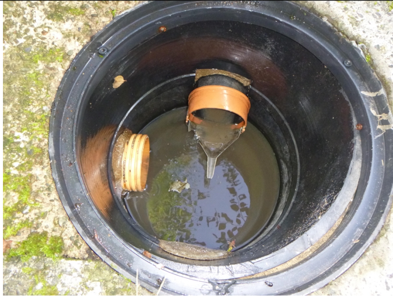
Photograph 2: Final effluent sample point
