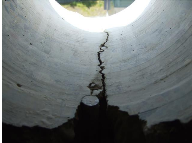
Figure 37: Photograph of cored hole through Boiler Box 3 west wall showing crack (pre-repair)
