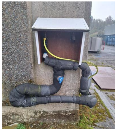
Figure 24: 2no. existing taps located at NE corner of RB2
