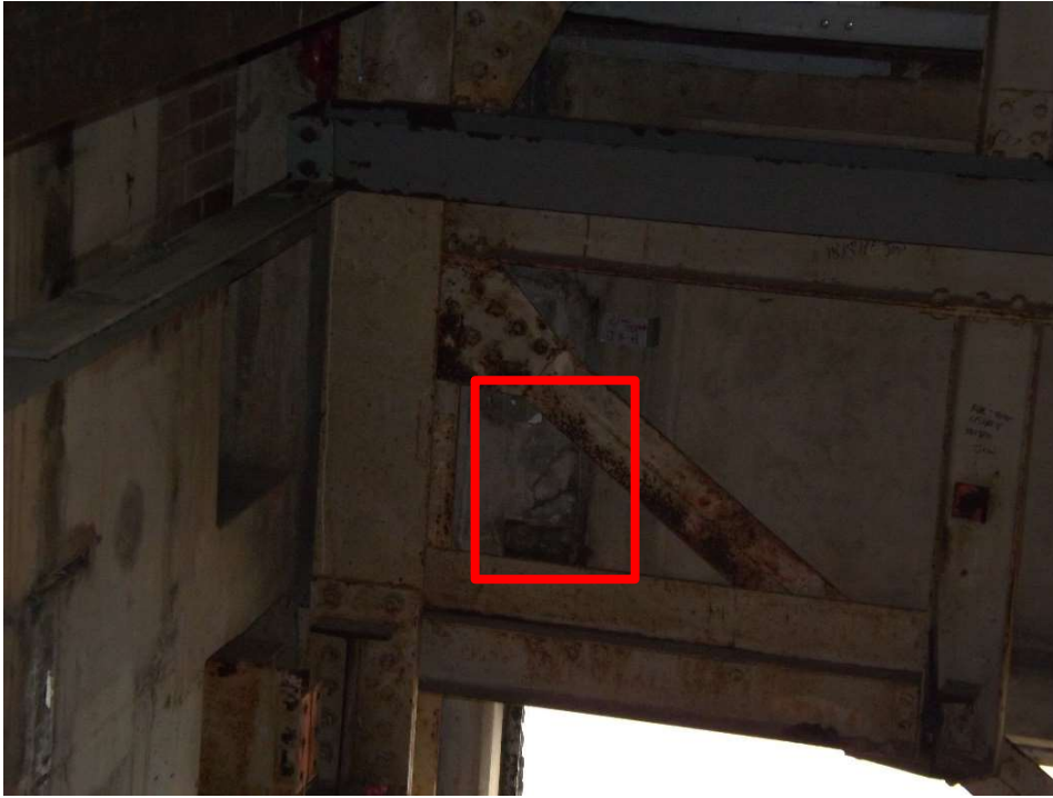
Figure 13: Class D Defect – 10314a/1
