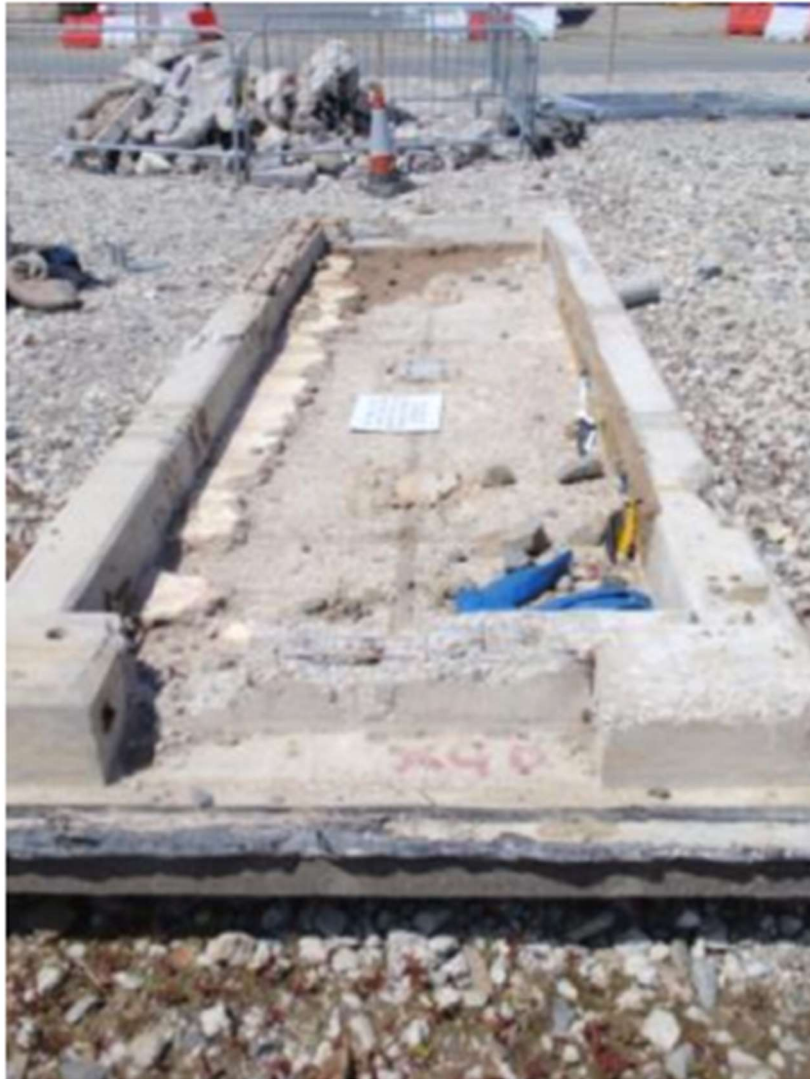
Figure 12: Defect panel W-0520
