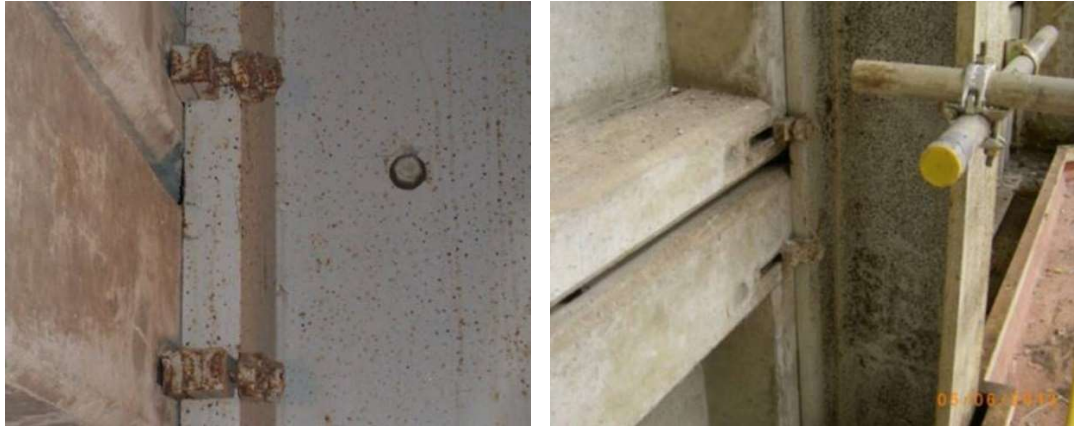
Figure 14: Lindaptor and Channel Support System Configuration (Connection to Column)
