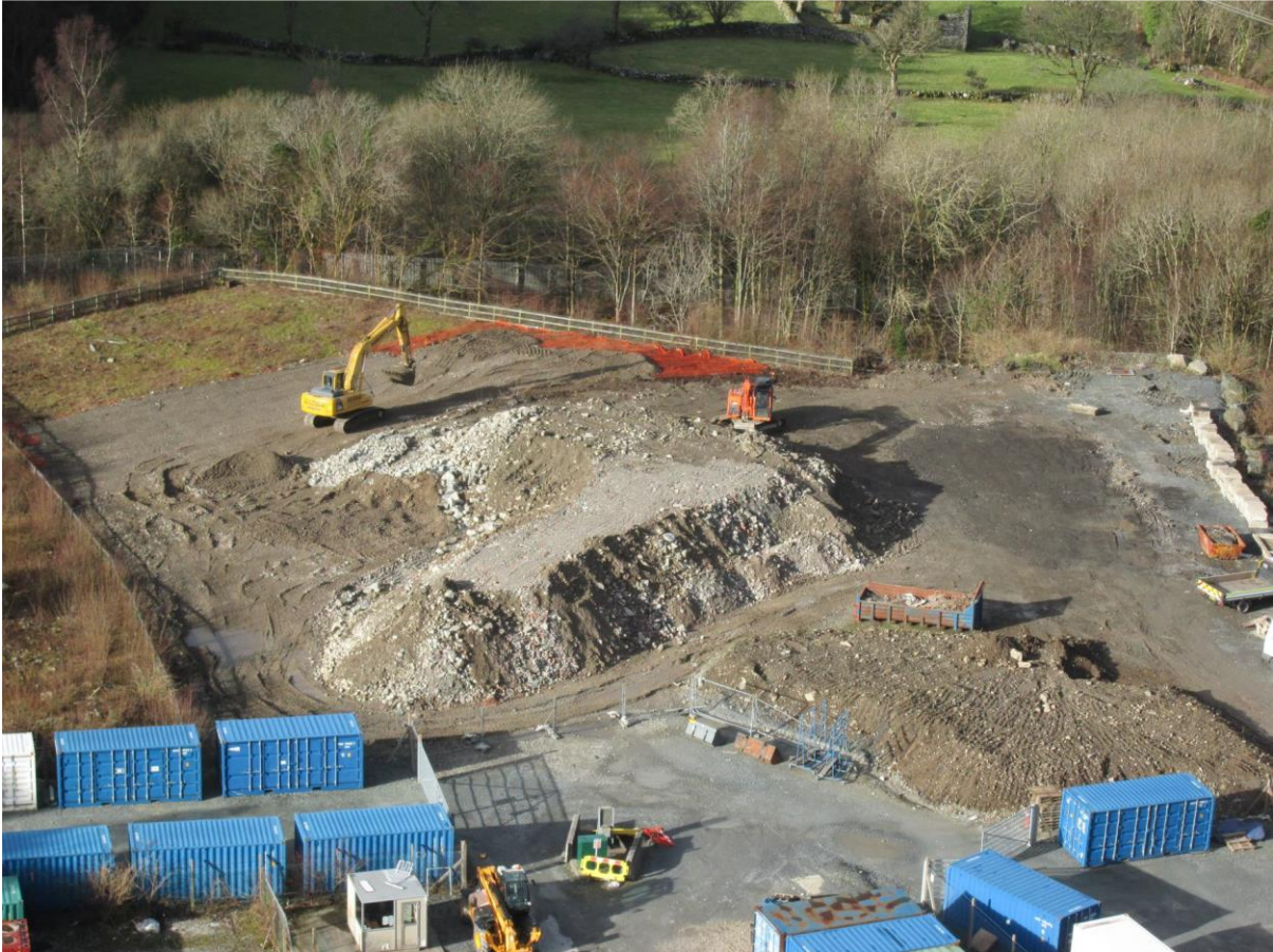
Figure 9 - Work to construct the original RCA laydown area (which now requires extension and improvement)
