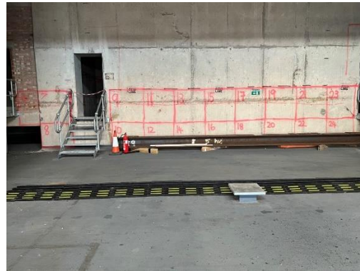
Shield Cooling Fan Room with grids
