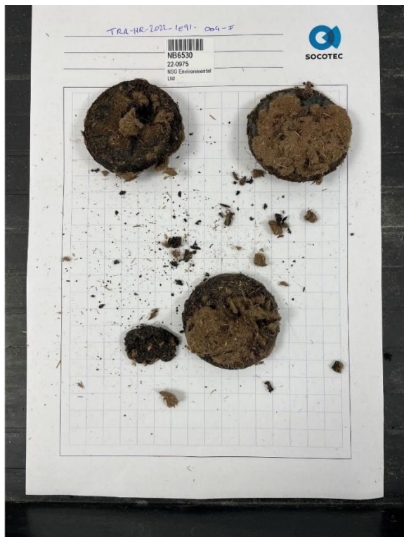
Roofing felt samples illustrating the mixture of the original felt (black) and insulation materials (brown)
