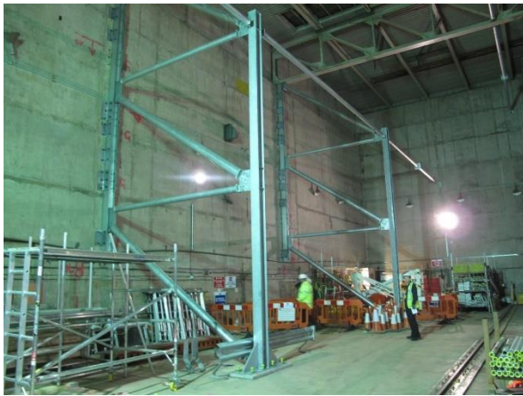
Top Duct Area
