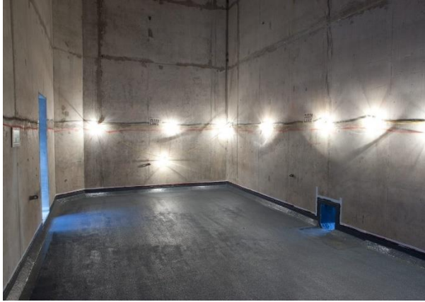
Hot Gas Duct Cell
