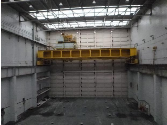
Charge Hall including crane and gantry
