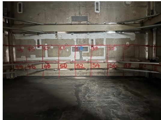
Boiler Box with grids
