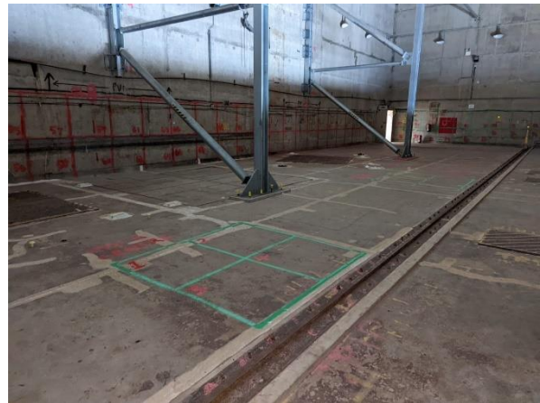
Top Duct Area with grids
