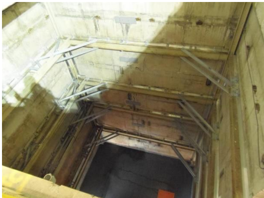
Boiler Box viewed from above
