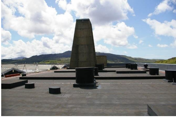
Reactor roof indicating Shield Cooling Stack
