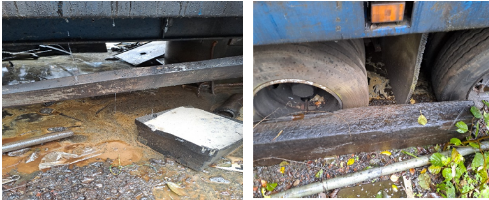
Photos 3 & 4 showing drip tray underneath the crusher
