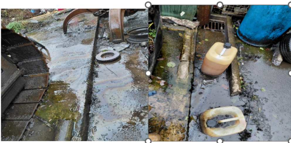
Photos 1 & 2 showing the raised pavement damaged
