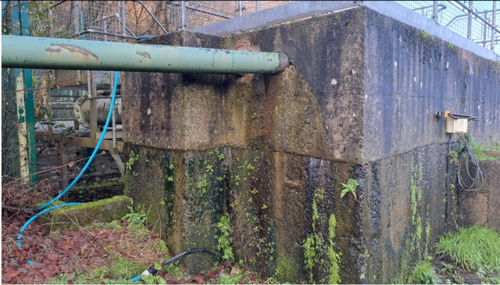
Figure 1 Leak from crack in the concrete of the inlet balance chamber
