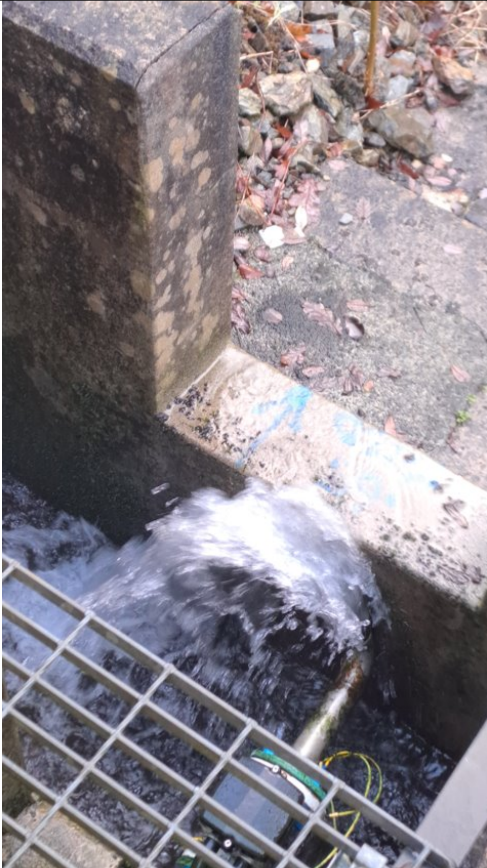
Figure 1 Flow from final effluent pipe splashing up and out of the final effluent sample chamber.
