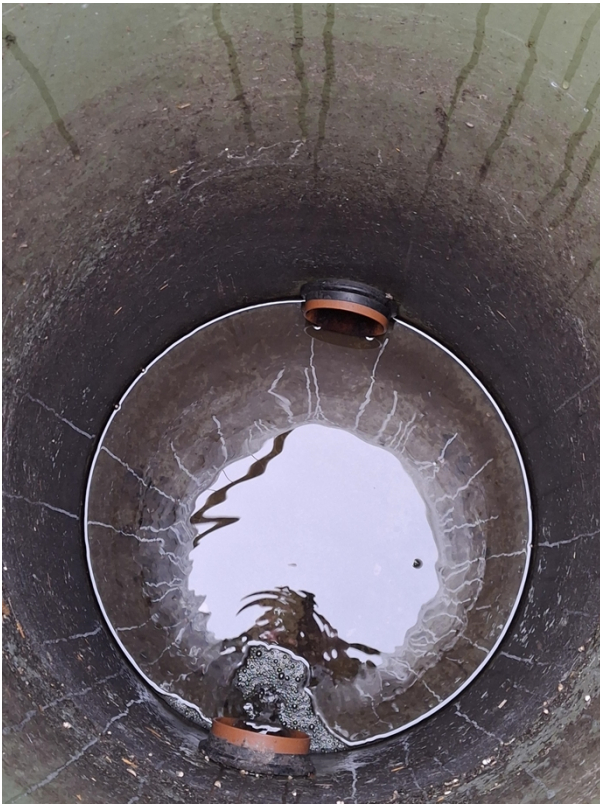
Fig2: Inspection chamber of system one
