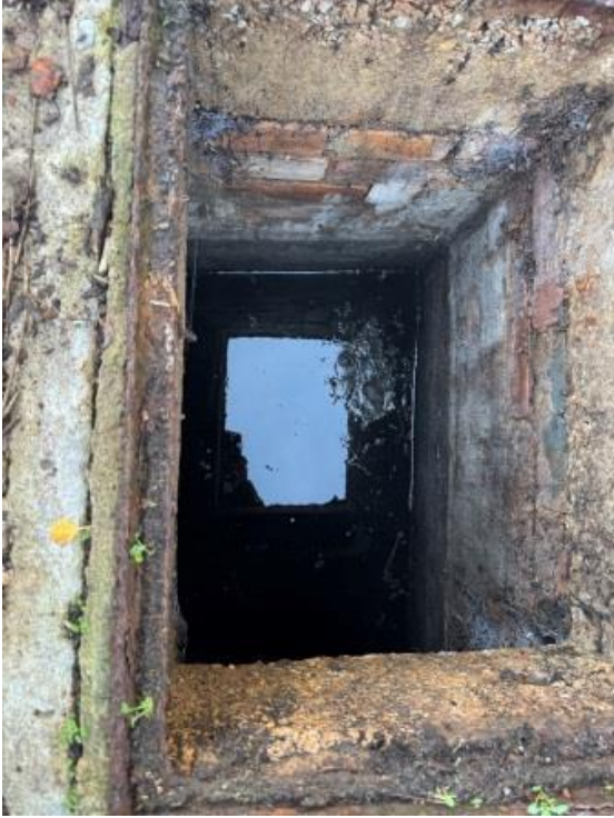
Pic 3 Picture of Water inside Cesspit Tank (Signs of water ingress)
