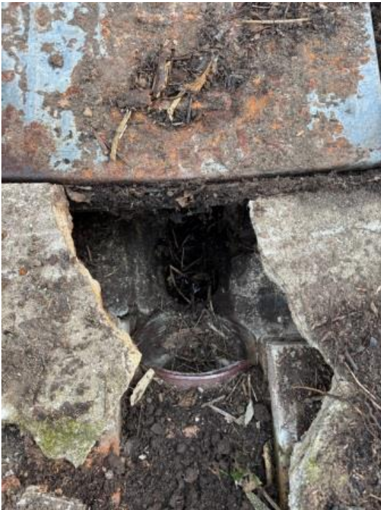
Pic 4 Inlet Pipework to Cesspit Tank
